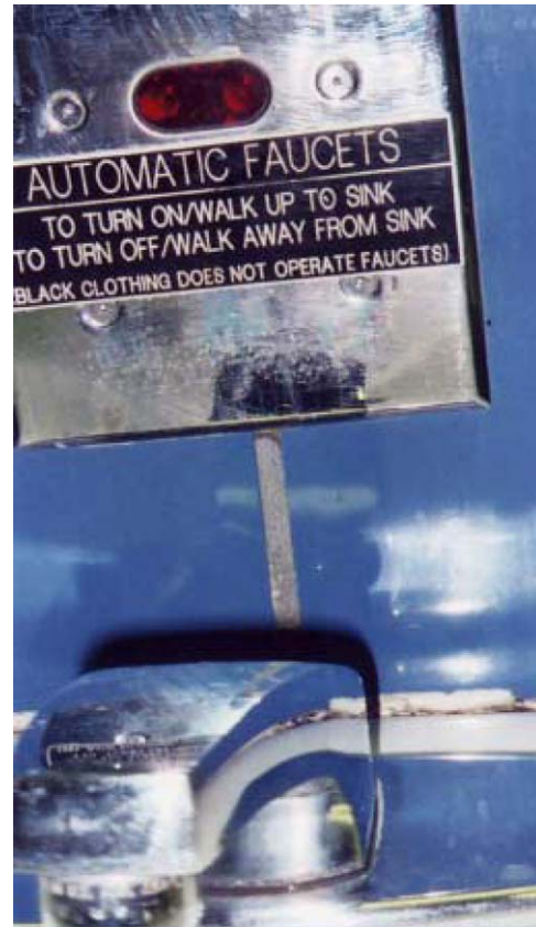
Fig. 1. Sign in the restrooms at Cincinnati airport.
