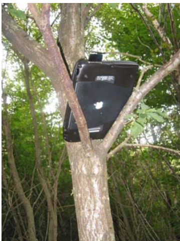
Figure 7: Network access point
